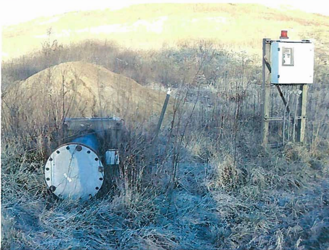
Date: 12/12/2011 Time: 7:54 a.m. Direction: north Photo by: Garrison Gross Exposure #: 018 Comments: riser pipe
